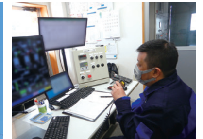
Monitoring in the control room
